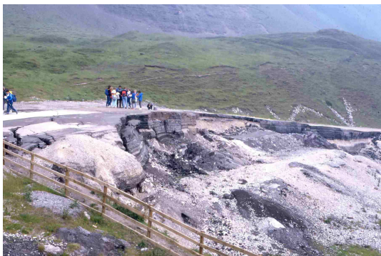
Mam Tor – the old road, now badly broken by landslide, and impassable since 1977. ( Photos: Peter Kennett )
