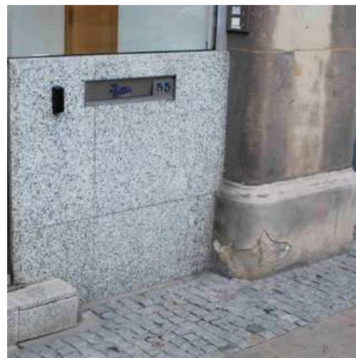
2. Facing stones made of grey granite and sandstone, Halifax Bank, Sheffield. (Photos: Peter Kennett)
