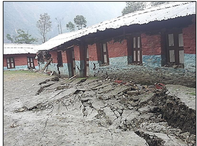
A school damaged by an earthquake.
