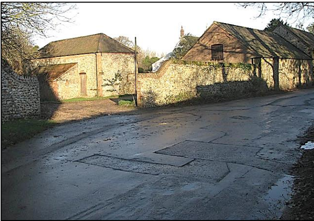
Patched road outside a farm house – which tarmac was laid first?
