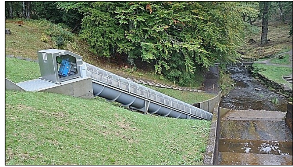
A new 17m long Archimedes screw installed at Cragside (file licensed under the Creative Commons Attribution-Share Alike 4.0 International license)
